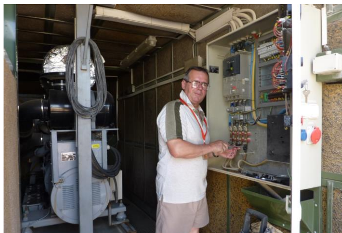
Fig. 1 Electric source plant MP-250, P_n = 200 kW (ISAF military mission in Afghanistan)
